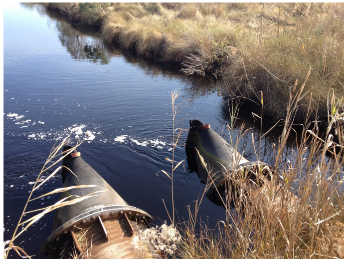
These water control valves allow freshwater to flow downstream but limit saltwater inflow upstream, protecting sensitive plant and animal species in the refuge.
